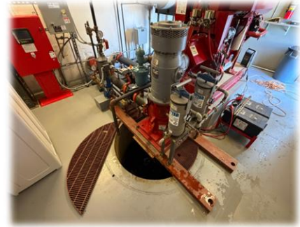
Pump station protection
