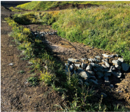
Figure 52 - Check dams or runoff "speed bumps" that have captured sediment. "Slow-the-Flow" BMPs require regular maintenance to keep them effective and to make sure they have enough capacity for sedimentation to occur. (Photo credit: John Teravskis)
